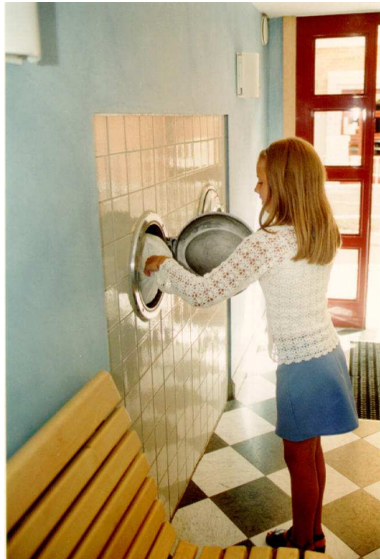
Picture 2: waste inlet located in the entrance hall of a building.
